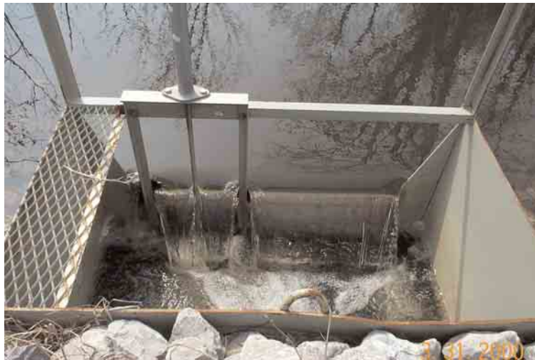
Water Control Structure functioning to restore natural water regime (note: spring run off being passed successfully).
